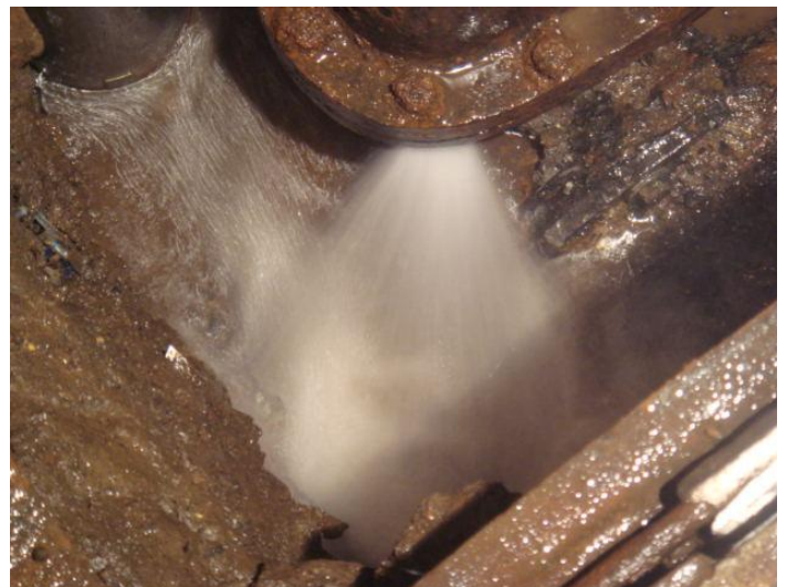
HIGH PRESSURE, CAST IRON VALVE LEAKING
