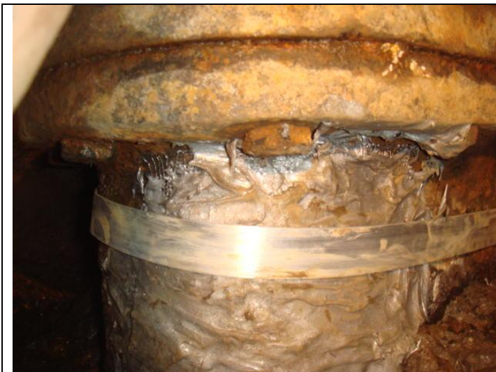
STEP 4 (A): ALUMINUM STRIP IS USED TO SECURE THE COLD WELDING COATING
