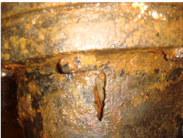
CRACK DETECTED AT THE HOUSING VALVE
