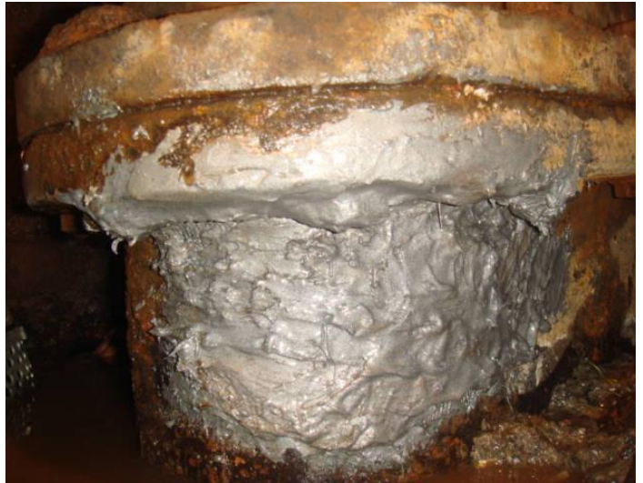
STEP 3: WIRE MESH IS COVERED WITH A SECOND COATING OF ECOPOWER'S COLD WELDING MATERIAL
